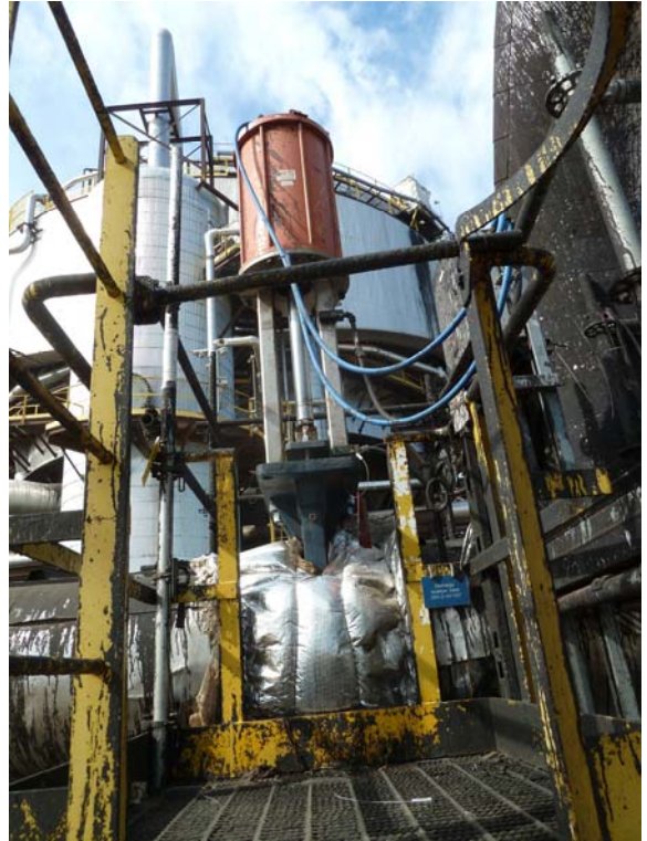
Pump isolation valve on floatation line.
