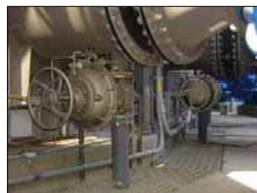
A 6" PVDF coated automated diaphragm valve on an absorber recycle pump drain line.
