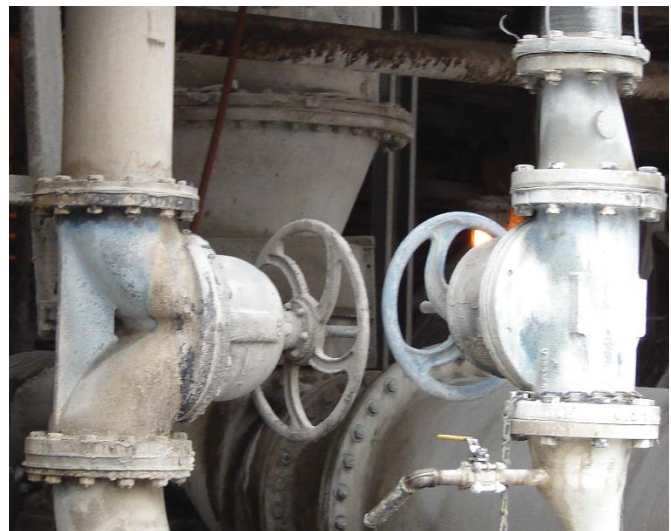
Weir type valve in Phosphoric acid service.
