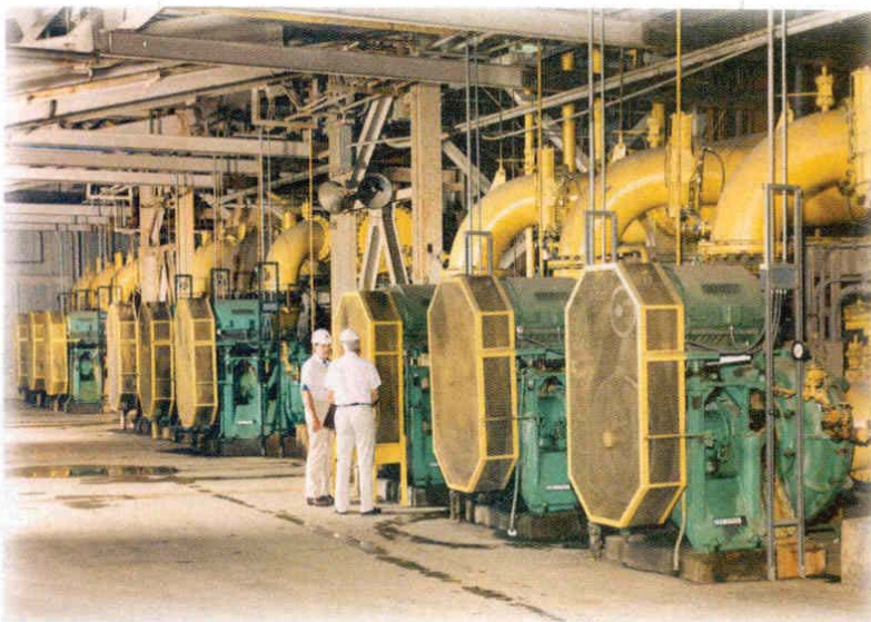
A bank of ITT rubber lined slurry pumps on FGD service at a Missouri power plant.
