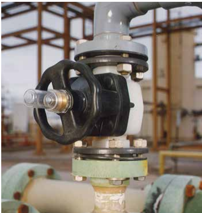
Solid Plastic Weir Type Valve on Acid Service
