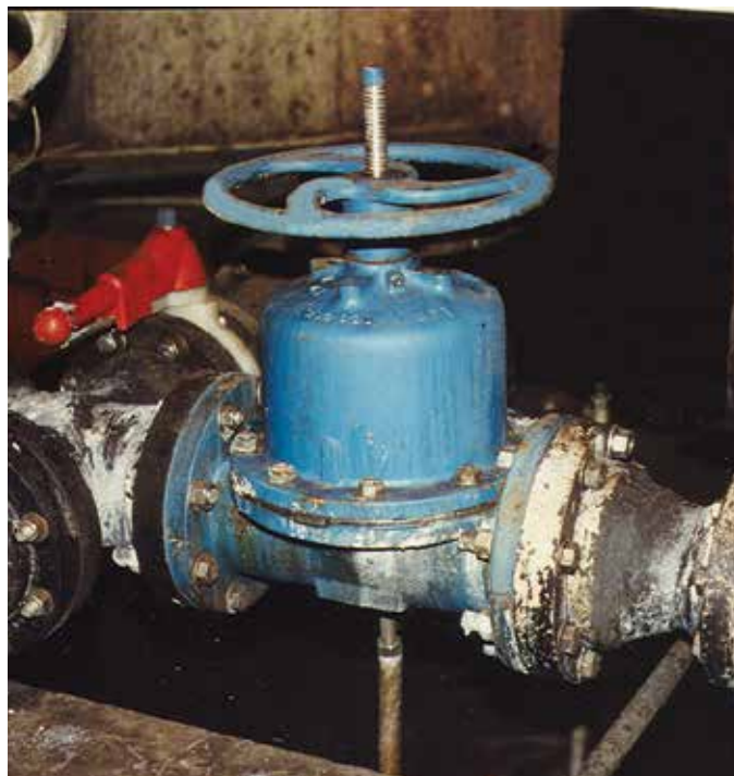
Straightway Valve on Abrasive Slurry Service
