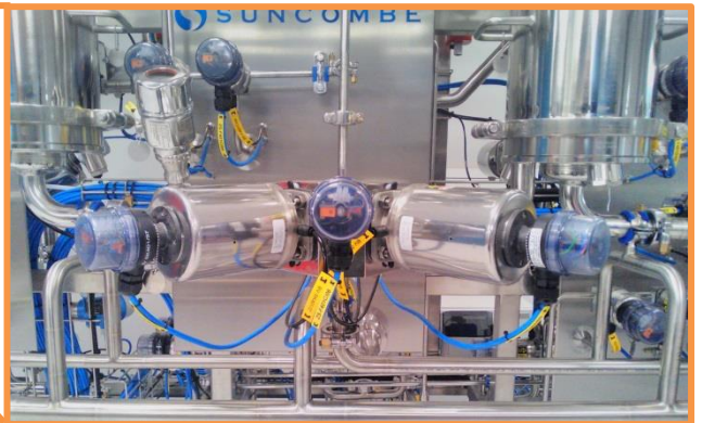
Pure-Flo block and bleed valve used on front of the filtration skid
