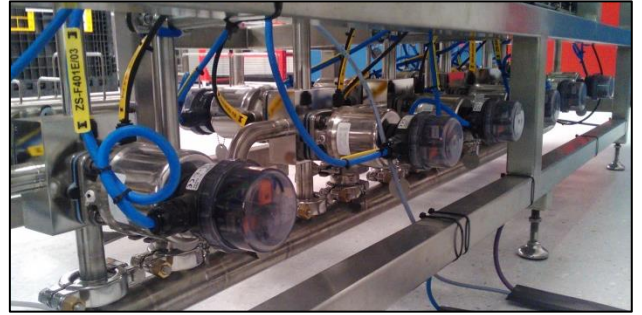
Row of Pure-Flo block body valves on the bottom of the filtration skid
